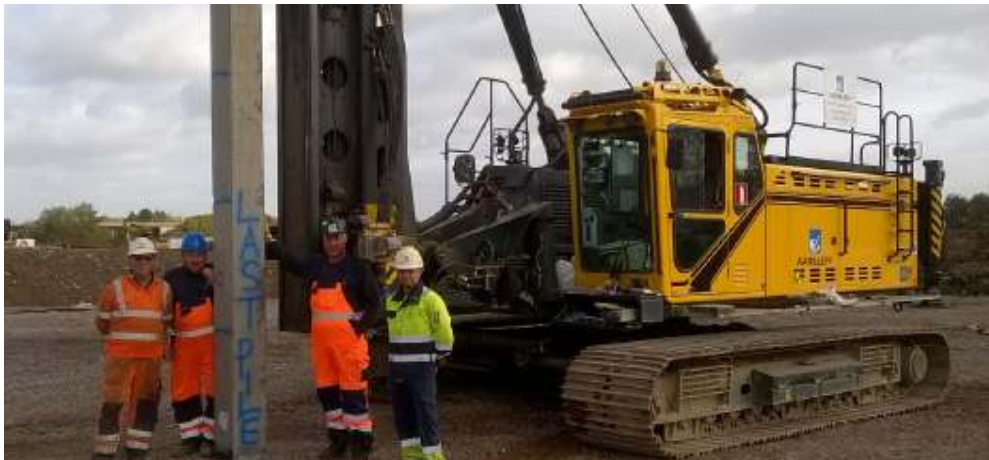
Last pile at Plot 4, Avonmouth (From Left: Andy, Toby, Rich, Wayne )- Richard Judd
